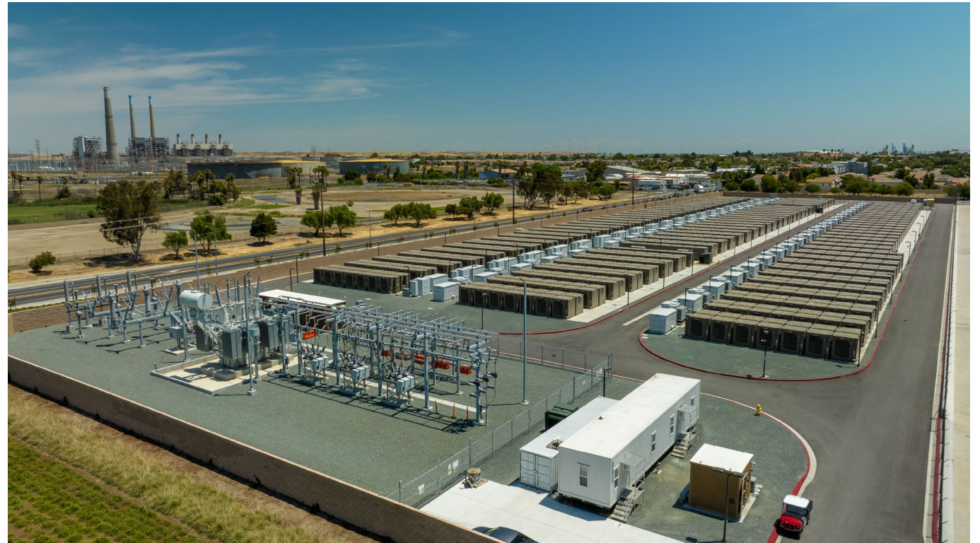
REV Renewables, 200 MW, Diablo Energy Storage project, Pittsburg, CA
