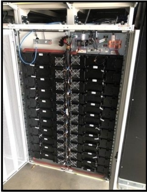
Figure 1-4: Example of battery rack with modules
